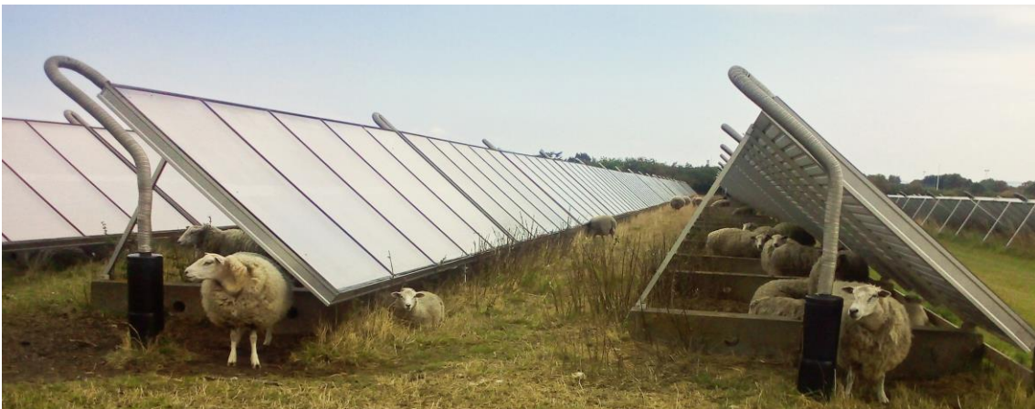
Figure 2: Solar thermal collector field of the SDH system in Marstal (DK).
