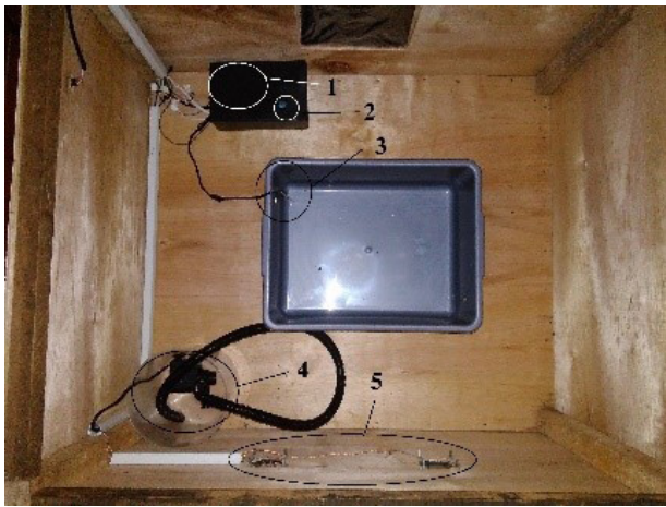
FIGURE 7. Electrical components in hydroponic grow room
