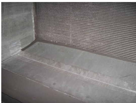
Figure 3.5. Duct floor upstream of heat exchanger after first fouling period in test 2B.
