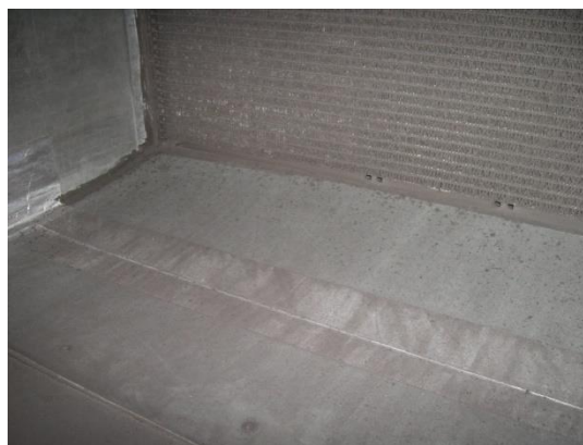
Figure 3.6. Duct floor upstream of heat exchanger after sixth fouling period in test 2B.
