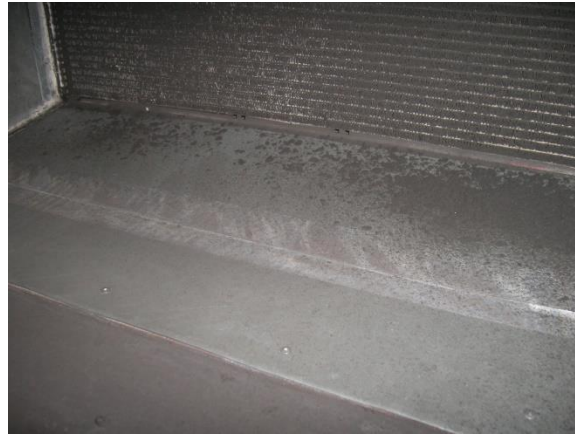
Figure 3.7. Duct floor upstream of heat exchanger after sixth fouling period in test 2C.
