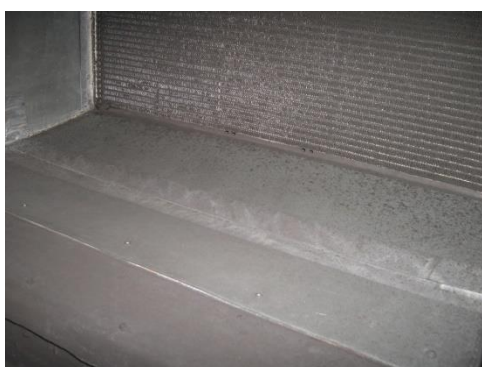
Figure 3.29. Test run 2E; higher pressure drop measured (2014).
