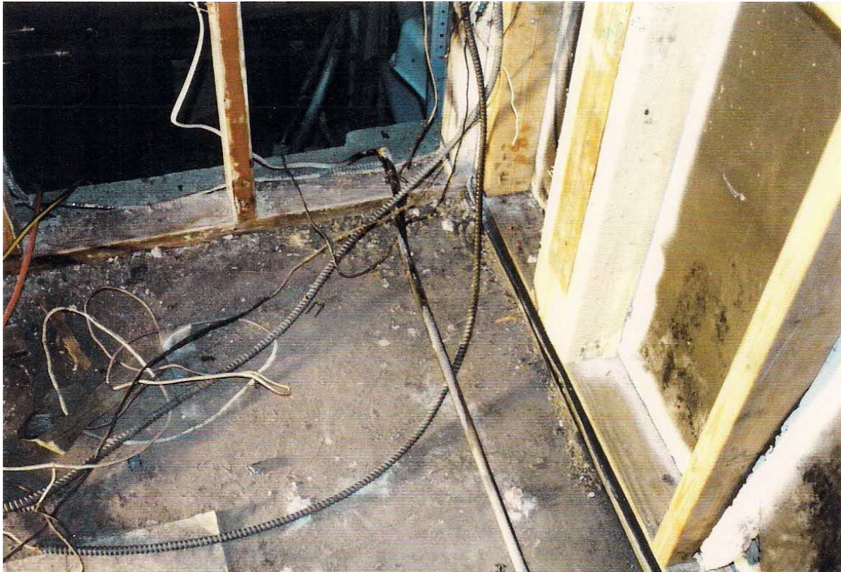
Figure 5: Fridge wire (long straight wire) was found as the point of ignition for the kitchen fire.
