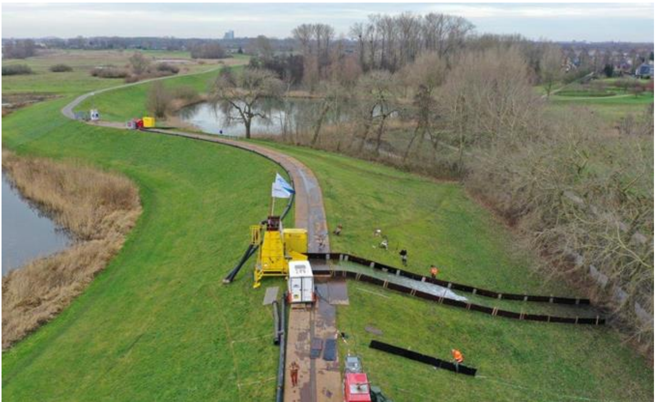
Figure 7: General set-up of the wave overtopping tests at the IJssel dike near Zwolle to establish the strength of grass covers on a sand dike. The upper left corner shows the frequency controlled pump and the pond where water was taken from.
