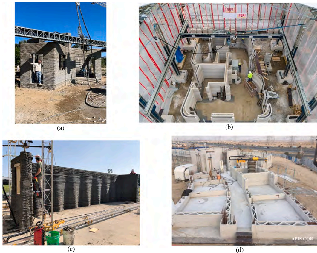
Fig. 6. a–d. On-site printing. (a) Holstebro (credit: COBOD International) and (b) Beckum Houses, both with a larger-than-building BOD2 printer, on one position. (c) B-Hut with a gantry on 2 subsequent positions. (d) Dubai office with cylindrical robot, on 12 positions.
