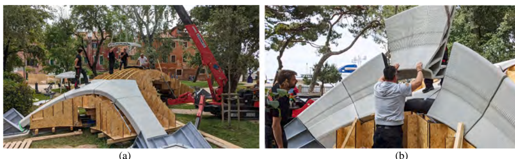
Fig. 7. a, b. Assembly of the Striatus Bridge. The elements were found to have sufficiently accurate dimensions to be placed without additional adjustments.
