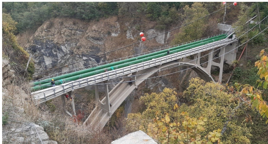
Figure 1. A view of the penstock bridge over the Dora di Rhêmes canyon, Introd (AO), Italy.
