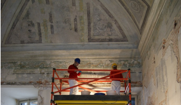
Figure 5: Conservative restoration performed on the decorative apparatus of the “room of frescoes”. Source: “Milano nei cantieri dell’arte”. Photographs by Alberto Favara / Villa Archive.
