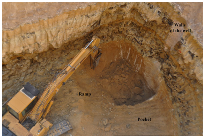
FIG. 2—Picture showing the pocket depository platform made by tracked excavator, next to the well shaft where fill can be placed.
