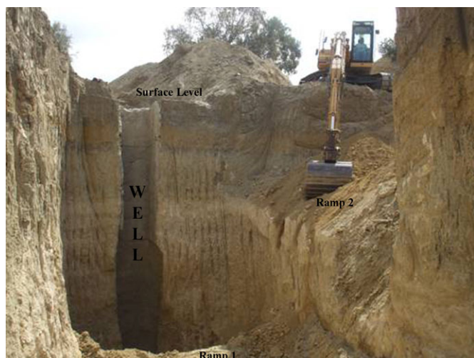
FIG. 4—Double-ramp method that was created to cope with the continuous flow of water of the well at Gokhan-Voni Village, in the northern part of Cyprus (2008).
