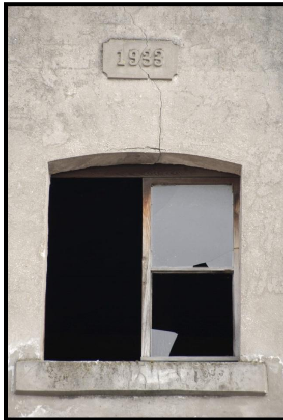
Figure 5.13. Factory Window Remains Example – Before Reevaluation 37
