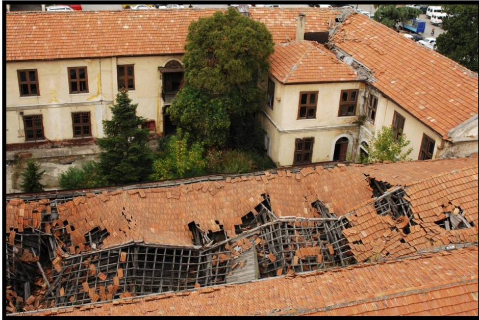
Figure 5.12. Ruined Factory Roof Before Re-evaluation 36
