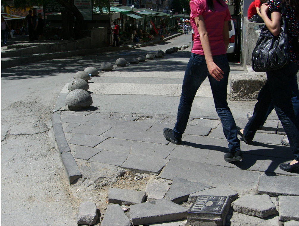
Figure 12.10. Distorted and broken sidewalks and pavements
