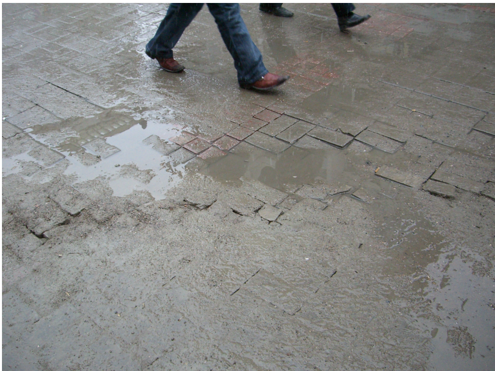
Figure 12.9. Distorted and broken sidewalks with accumulated rain water (January, 2009 weekend afternoon)
