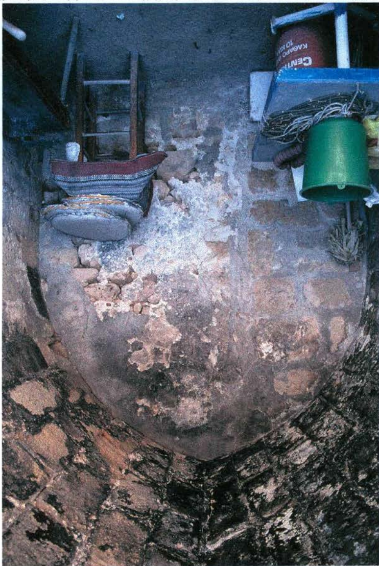
27 Detail of arched room in the building on Paphias Aphroditis Street (photograph by the author)
