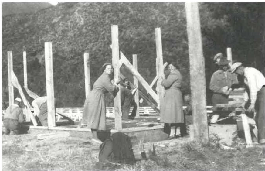
Building the Finnish sauna in Kawerau in 1955. Notice women also involved in the work. SI, Turku.
