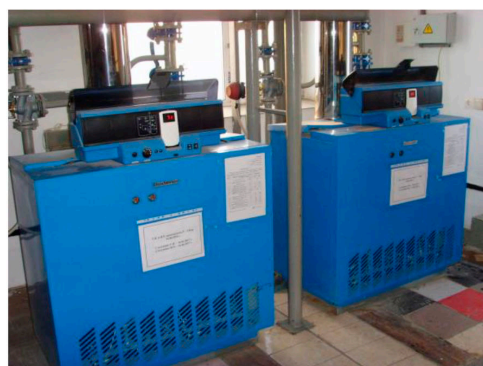
b) hot water boilers of the heating system circuit
