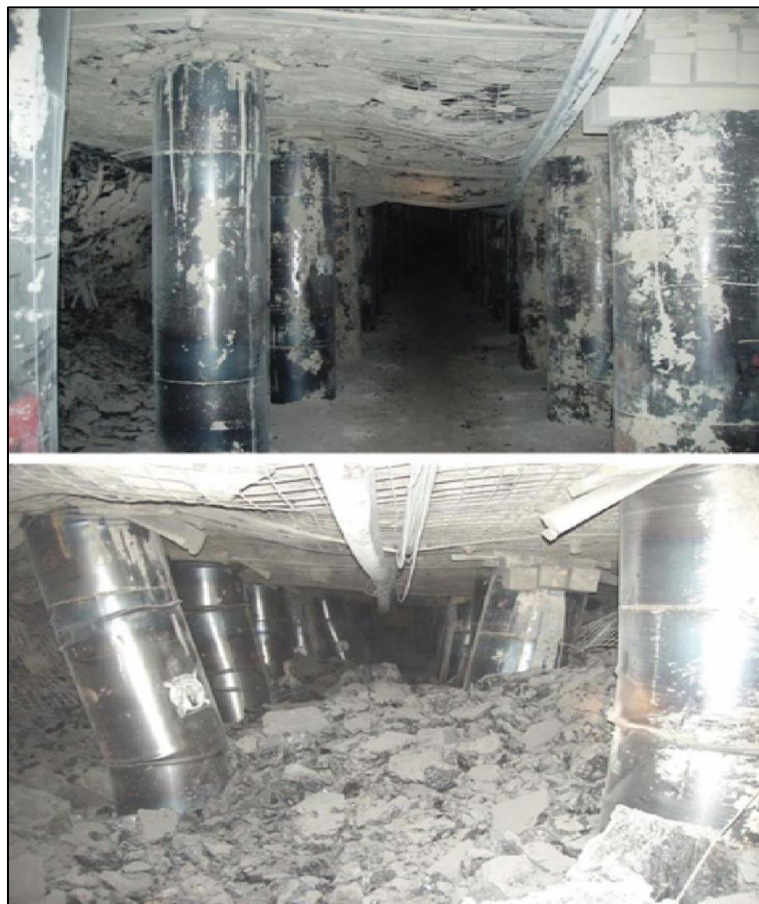
Figure 2: Effect of a coal burst on a gateroad before (top) and after (below) (Mark from an unspecified US mine in the North Fork Valley, 2016)
