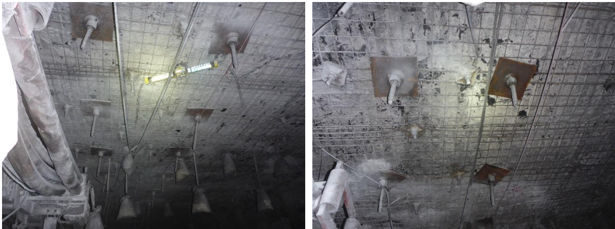
Figure 7: Photos of 70 t Sumo reinforced with Booster cable installed underground at Dendrobium
