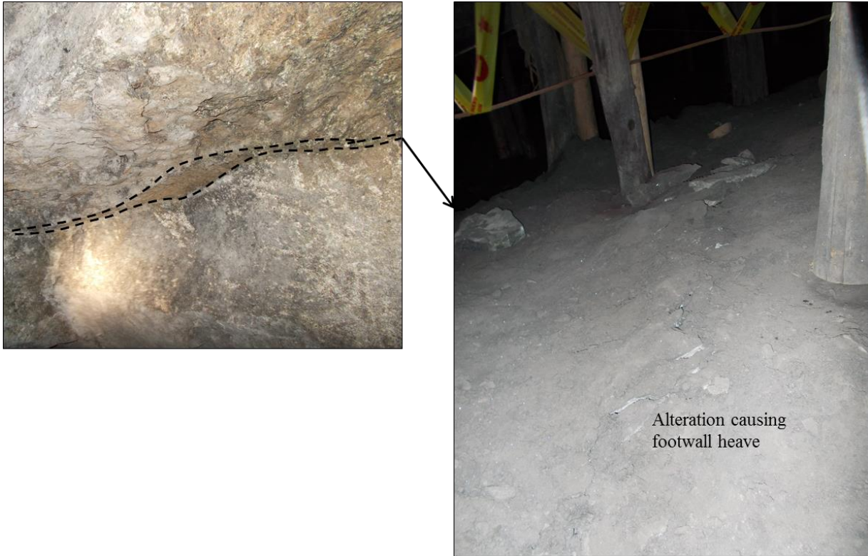
Figure 4.8: An alteration zone along the footwall contact of the UG2 Reef causing footwall heave and premature failure of the installed timber elongates. This can result in large-scale hangingwall failure.
