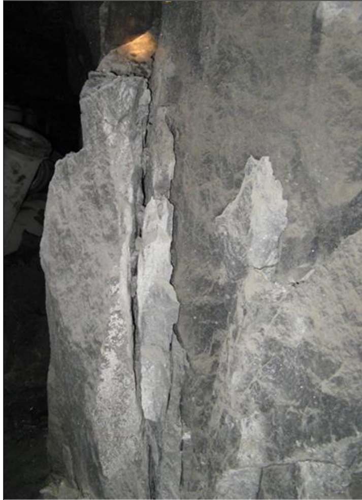
Figure 2.30: Slabbing noted at the edge of a pillar. The slabs are defined by joint planes which are mobilised by alteration zones along the pyroxenite and chromitite contacts (i.e. Figure 2.31).
