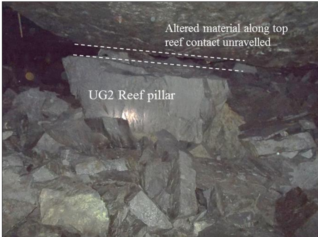
Figure 4.4: An alteration zone along the top reef contact affect the pillar strength and integrity.
