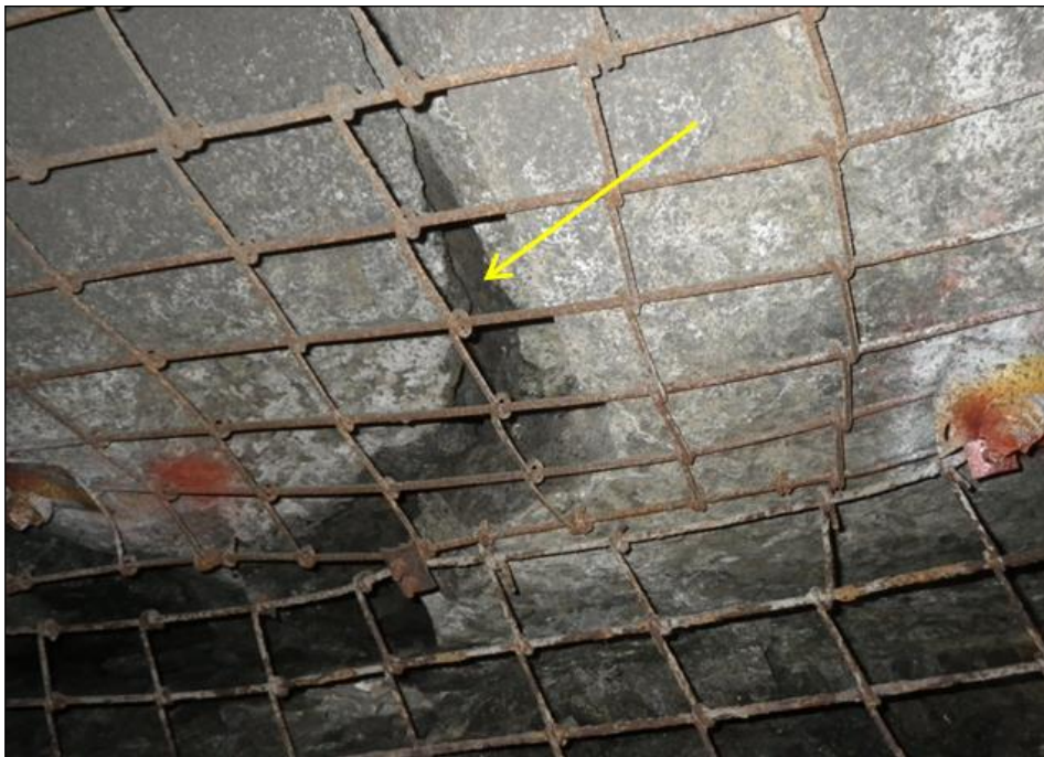
Figure 4.6: An alteration zone in the hangingwall can cause the unravelling of key blocks due to separation along joints or parting planes.
