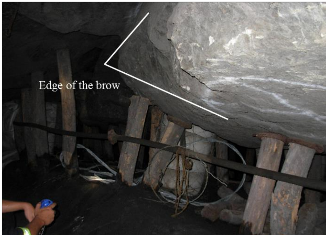
Figure 2.17: Buckling of timber elongates as identified during a 2009 study. The Marikana structure defines the edge of the brow.
