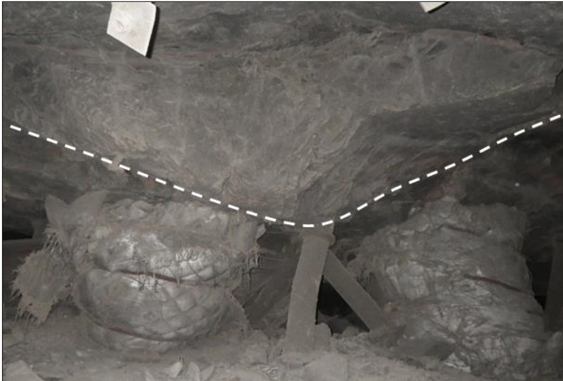
Figure 3.15: Failure of grout packs and timber elongates owing to excessive loading from probable separation along the hangingwall 1A / hangingwall 2 contact.
