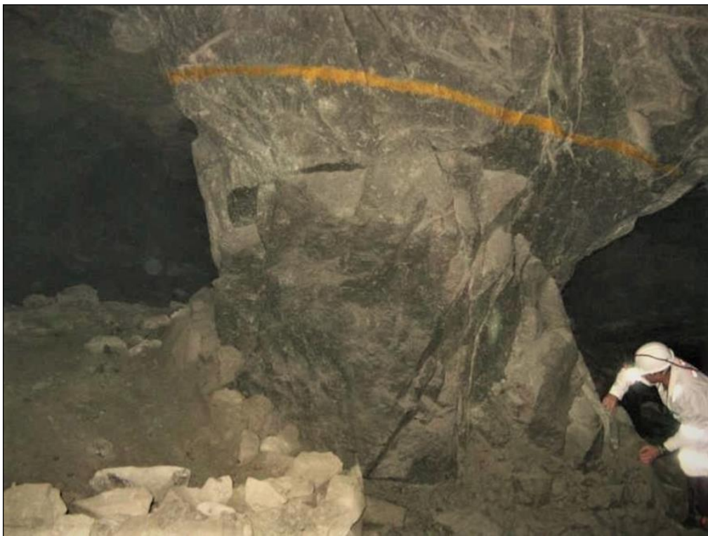
Figure 2.35: Unravelling caused by joint planes in the pillar (More O’Ferrall and Du Plessis, 2017).
