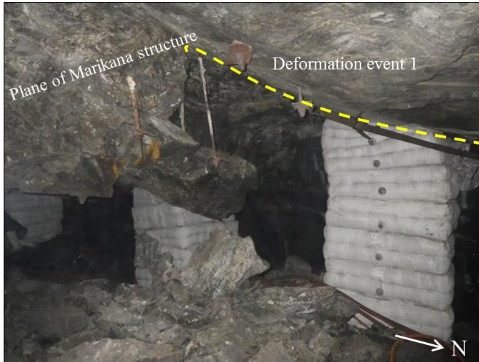
Figure 3.30: Intersection of deformation event 1 (ramp structure) and a Marikana structure. Alteration has also been exposed along the hangingwall pyroxenite units. This represents the worst case scenario and unfavourable conditions. Rock bolt support failure is also visible in the vicinity of the fall of ground.
