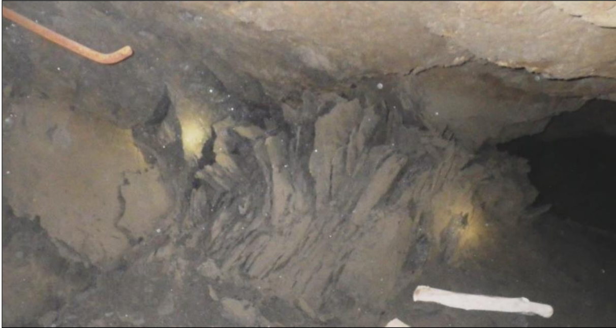
Figure 4.14: Anomalous pillar behaviour (illustrated in Figure 4.19) where stress fracturing was identified in the vicinity of the fall of ground where an alteration zone occurred along the top reef contact.
