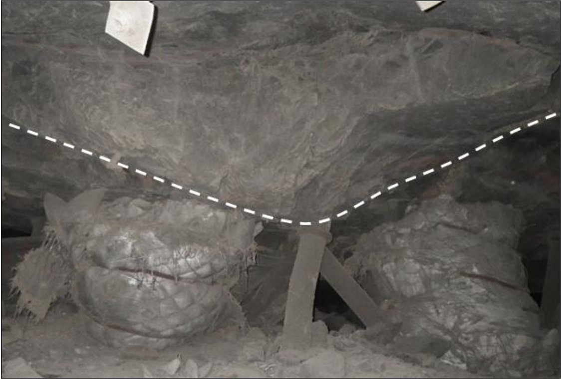
Figure 1.10: Large-scale instability showing the loading and failure of the support units. The support units were loaded as a result of separation along the hangingwall 1A/hangingwall 2 contact (12 – 15 m in the hangingwall). The peak support capacity for elongates are 27 t and for the 1.2 m diameter grout packs are approximately 500 t. The panel was abandoned and had to be re-established.
