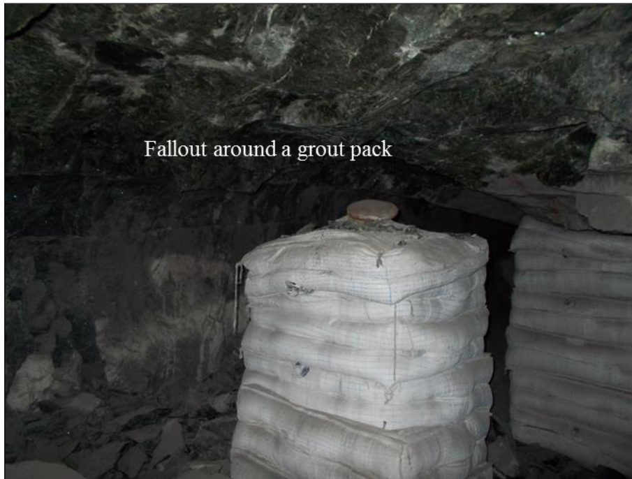
Figure 4.1: An alteration zone along the top contact of the UG2 Reef, causing fallout around an installed grout pack. This results in ineffective support being provided to the hangingwall which could result in large-scale unravelling, especially when intersected by prominent regional geologic structures as described in Chapter 3.
