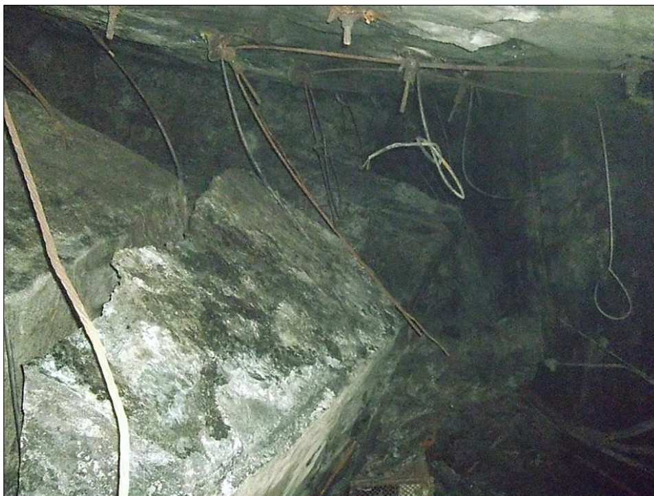
Figure 3.27: Collapse in a belt drive. It is suspected that the poor quality of cable anchor installation contributed to the collapse.
