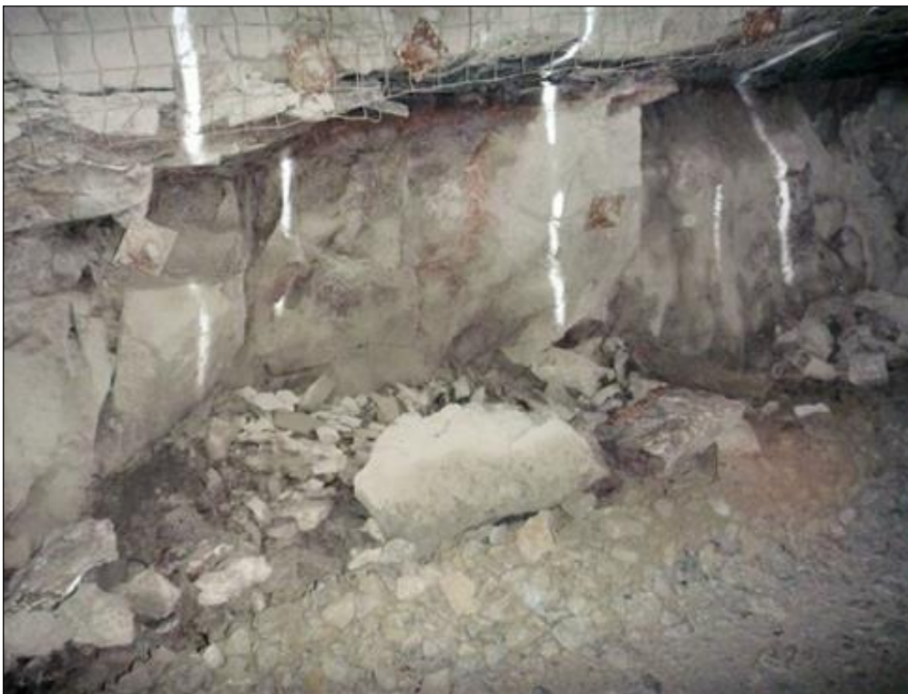
Figure 2.40: Unravelling of the pillar wall below the shear layer (More O'Ferrall and Du Plessis, 2017).
