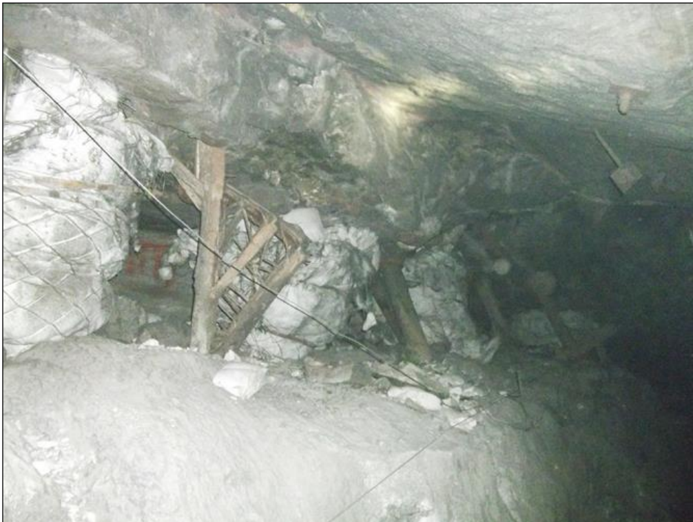
Figure 2.19: Fall of ground visible along a gully at Saffy Shaft where the support units failed when the hangingwall beam detached at a height of approximately 15 m at the hangingwall 1A/hangingwall 2 contact. This resulted in failed timber elongates and crushed grout packs.
