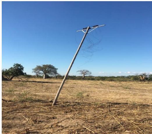
Figure 6: Damaged fixed telephone line in Binga Simatelele (2018)
