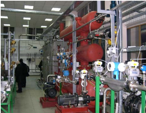
Figure 6 Three-phase test bench (GET195-2011) at VNIR, Kazan, Russia.
