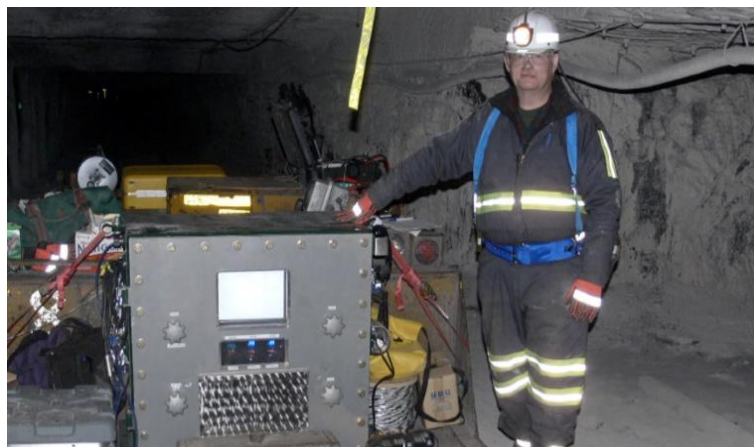
Figure 52: Underground transceiver units of the through the Earth MagneLink Magnetic Communication System (Lockheed Martin, 2017)
