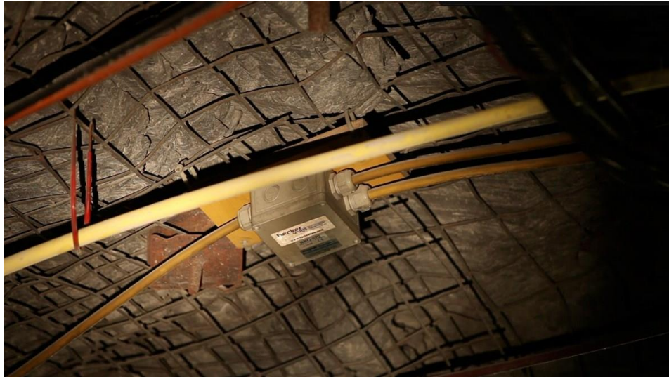
Figure 18: Amplifier of a leaky feeder system installed on the hangingwall of a mine haulage ( www.meglab.ca/en/products/wireless-communication/ , 2017)
