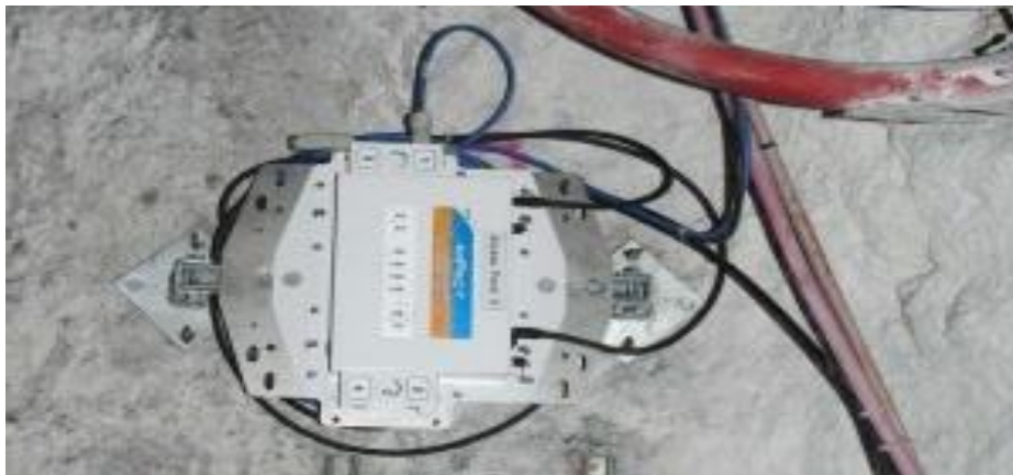
Figure 30: Wi-Fi access point installed in an underground mine to provide network coverage (Mine Site Technologies, 2017)
