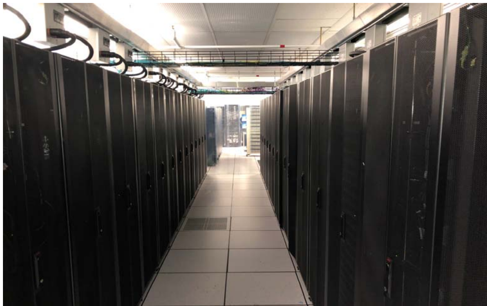
Heat from NPS computer racks is exhausted into a "hot aisle".
