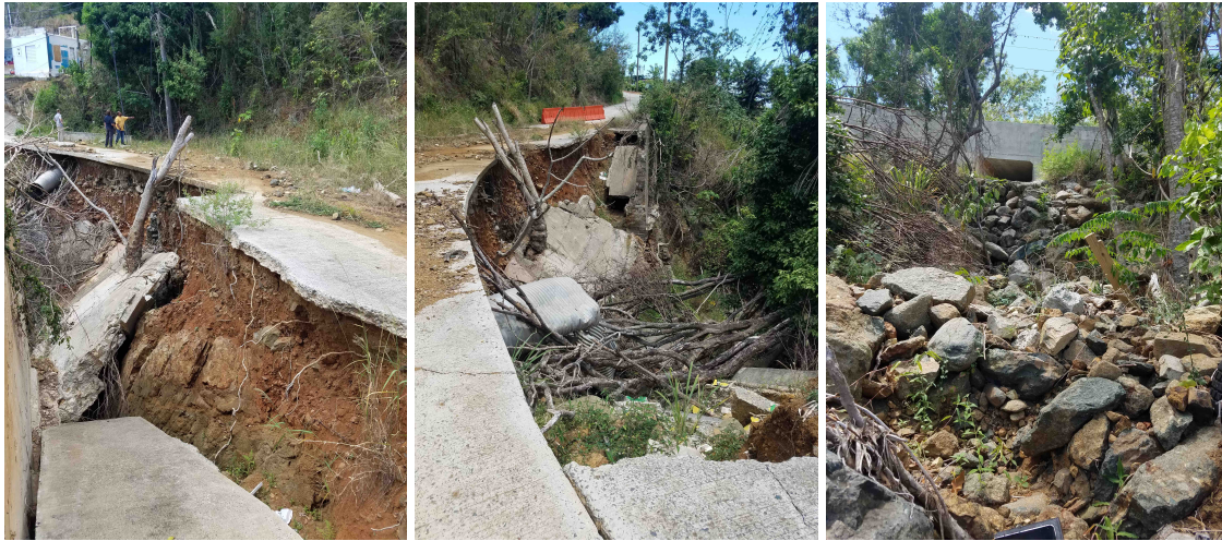
Figure 32. Left and Center: A washed out road and culvert on St. Thomas, as a result of Irma, still left in disrepair more than nine months after the hurricanes, June 2018. Right: A drainage culvert, part of the 'guts', on St. Thomas, remains full of debris.
