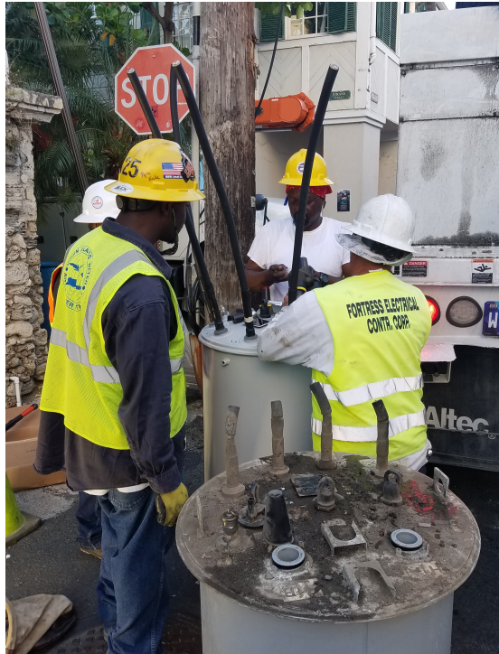
Figure 22. WAPA employees replace a blown underground transformer in downtown Christiansted. This outage lasted approximately 24 hours, affected numerous businesses and residents and, according to the repairmen, was the result of a faulty transformer. Photo: NPS, March 2018.
