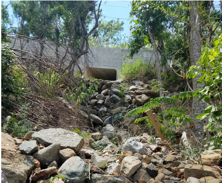
Figure 23. An uphill view of a drainage culvert and a 'Gut' line. Photo: NPS, June 2018
