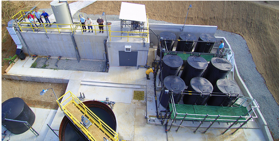
Figure 28. Bordeaux WWTP on the western side of STT. Source: Fluence Corporation (2018).
