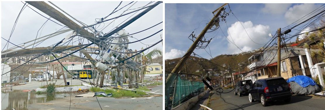
Figure 21. Downed and damaged power/telecommunications lines across the territory as a result of Hurricanes Irma and Maria. (Left) Damaged Power Lines STT. Photo: VI Consortium (Right) Damaged Power Lines Charlotte Amalie. Photo: Samoa Observer.
