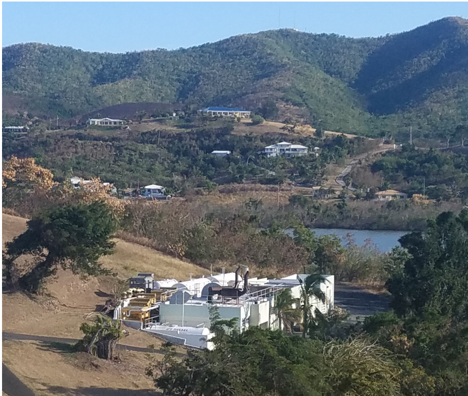
Figure 17. The Buccaneer Hotel operates independently from WAPA using their own diesel power generation site that reportedly maintained electrical power throughout Hurricane Maria. Photo: NPS, March 2018.
