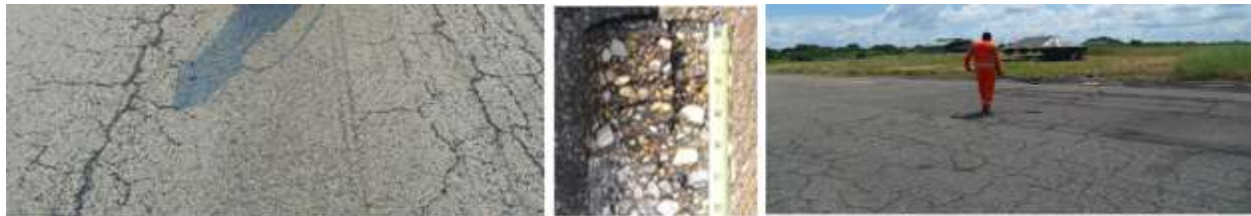
FIGURE 1 Example of an Old Cracked HMA Pavement.
