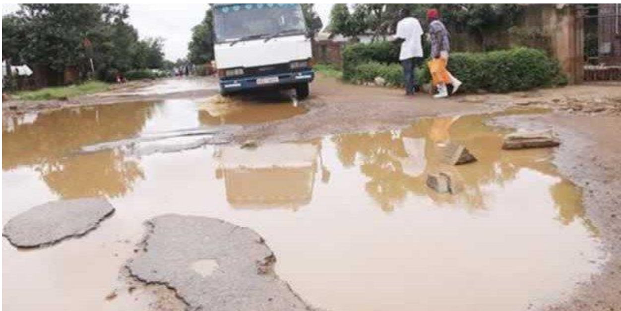
Plate 4.1: Some of the potholed roads in Southlea Park
