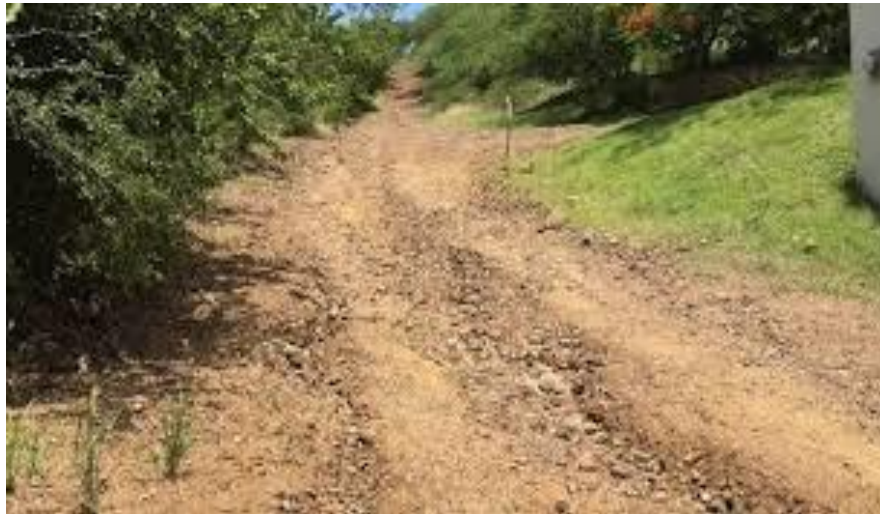
Figure 2 Excessive stoniness on unpaved roads (from Unpaved Road Standards for Caribbean and Pacific Islands', 2021).
