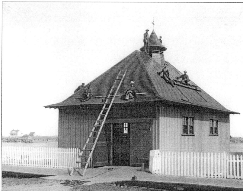
Figure 181. Surfmen Painting the Boathouse Roof, Coquille River Life-Saving Station, Circa 1900. Source: Bandon Historical Society.
