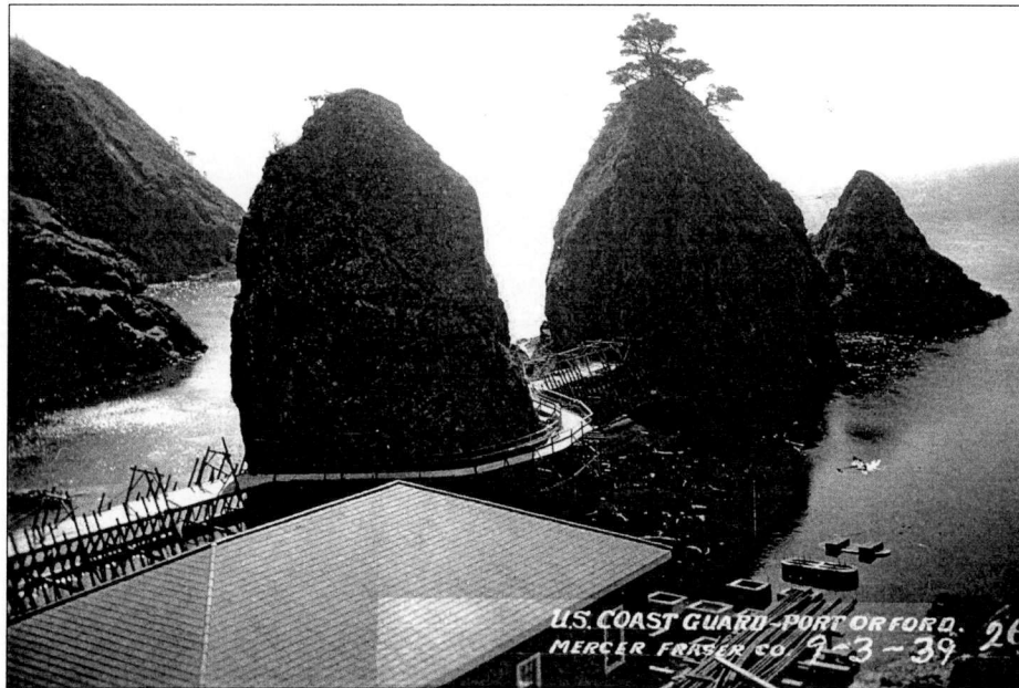
Figure 179. Boathouse Launchway and Breakwater Under Construction, 1939. Source: National Archives (RG 26-DS Box 21 Folder 437).
