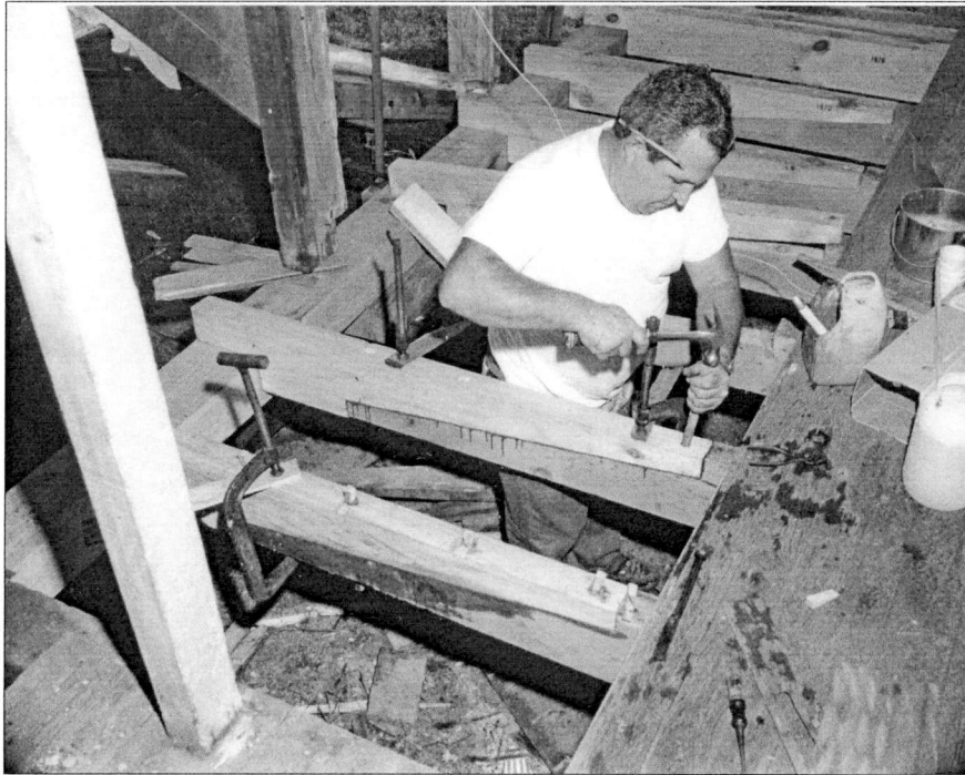
Figure 182. Splicing Floor Joists at Block Island Life-Saving Station, Rhode Island, 1970. Source: Mystic Seaport (#70-8-364).
