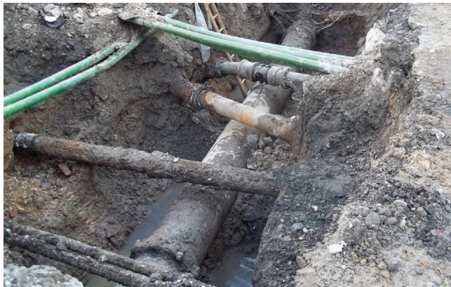
Figure 7. An exposed 20 in. (0.508 m) trunk main in situ at Regent Street in central London with several other pipes and services crossing it, showing the restricted space available around a main
