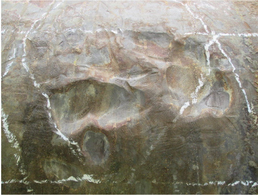
Figure 7.3 - Corrosion pit after the graphitic corrosion has been partially removed during surface preparation.
