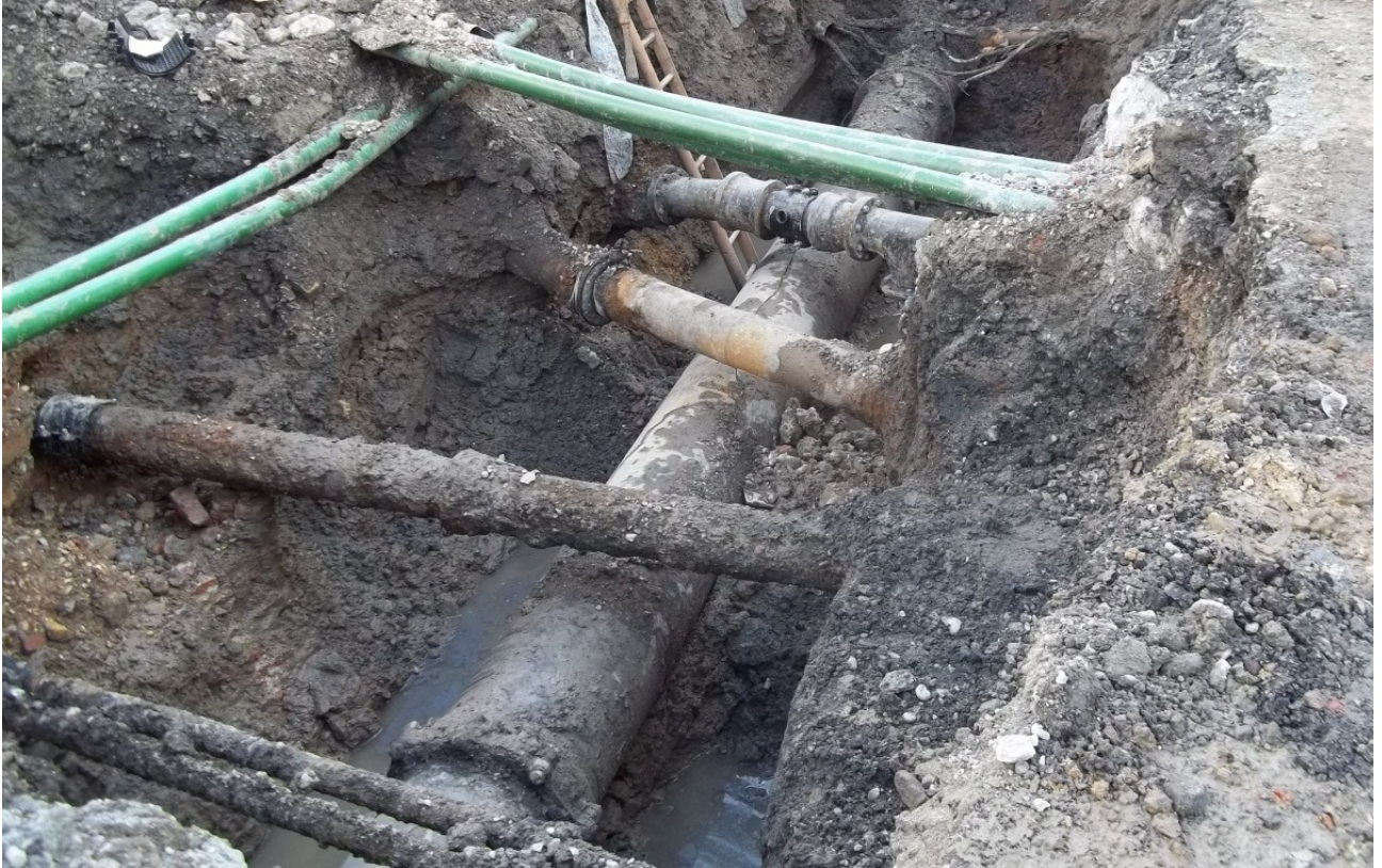
Figure 4.2 - Exposed 20" trunk main in situ at Regent Street in central London with several other pipes and services crossing it showing the restricted space available around a main.
