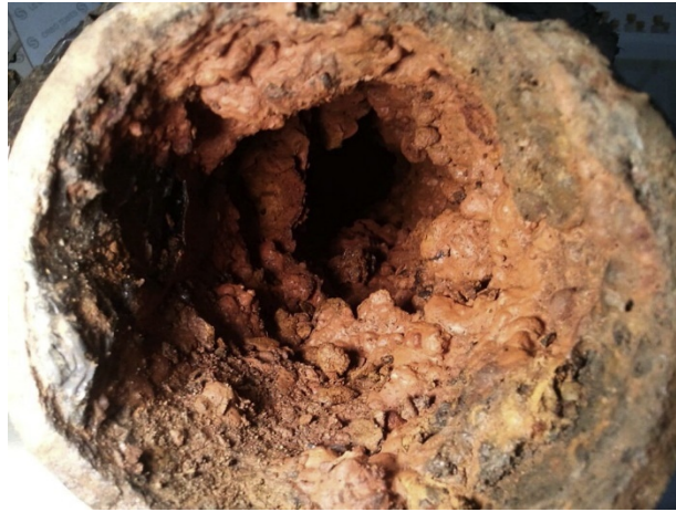
Figure 2.5 - A view of the inner surface of a water main showing significant tuberculation bubbles lining the whole inner surface of the pipe. After Świetlik et al. (2012).
