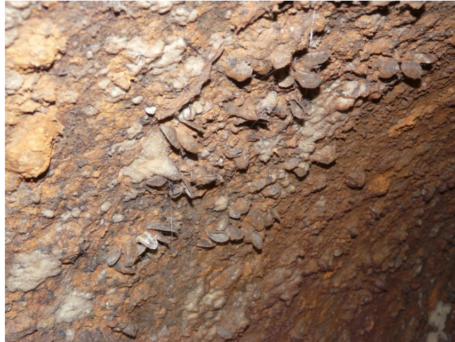
Figure 4.1 - Example of tuberculation build-up on the inner surface of a cast iron trunk main.
