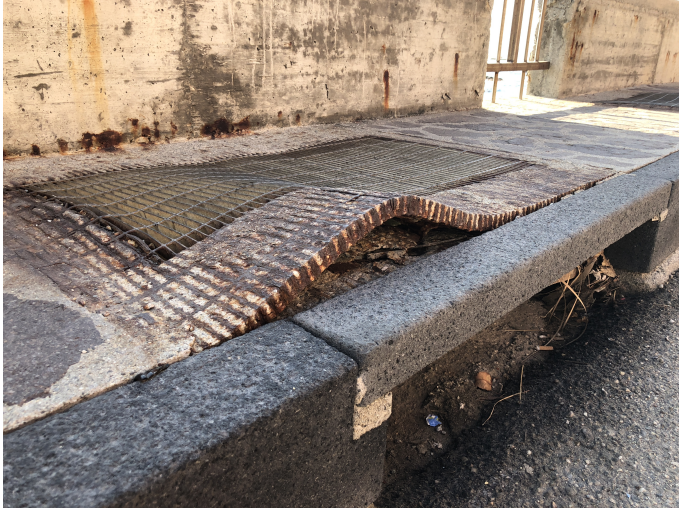
Figure 2: Buckling delamination of a sidewalk steel grid
