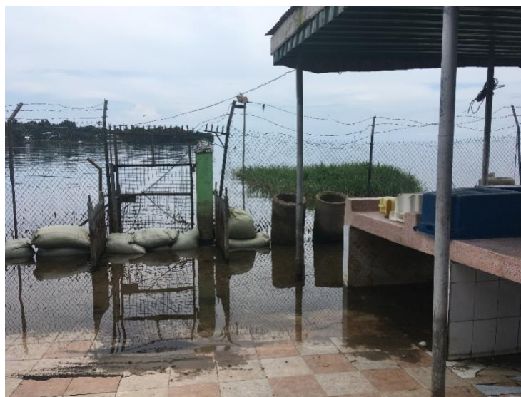
Figure 21: Flooded settlement at Nakatiba landing site
