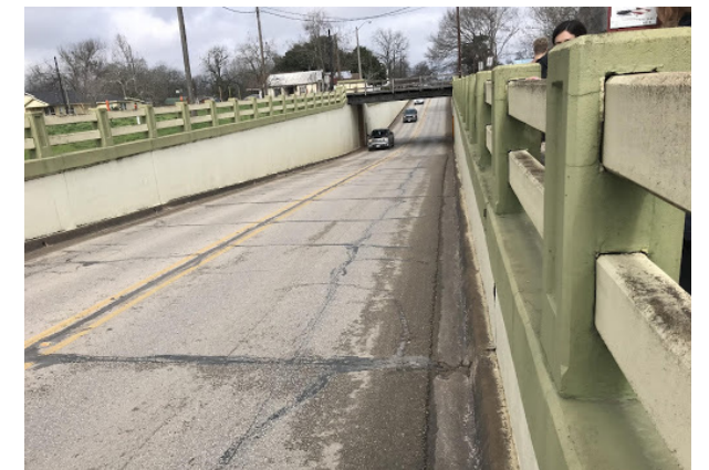
No pedestrian access to bridge crossway
