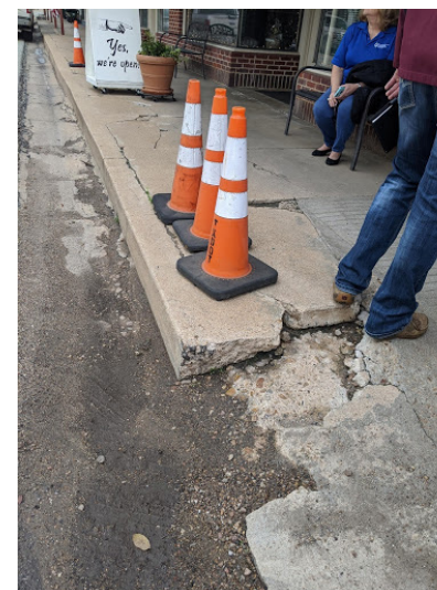
Poor Street Access
