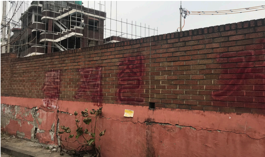
Figure 40. A brick wall with letters that say “Demolish” across the street from a high-rise mixed-use building, which provides a different landscape from the preservation happening in other parts of Seongsu. Image source: author, 2020.
