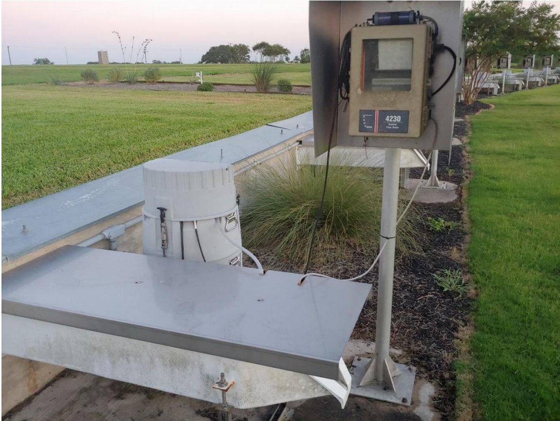
Figure 3.3: Teledyne ISCO flow meter and runoff sampler
