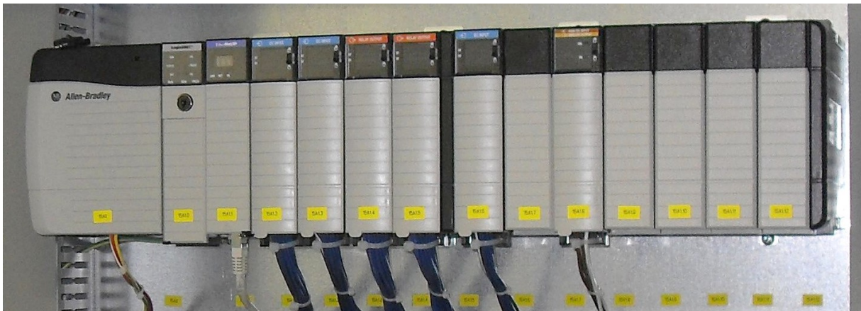
Figure 1-1 An Allen Bradley PLC Chassis Wired to a Control System [9]
