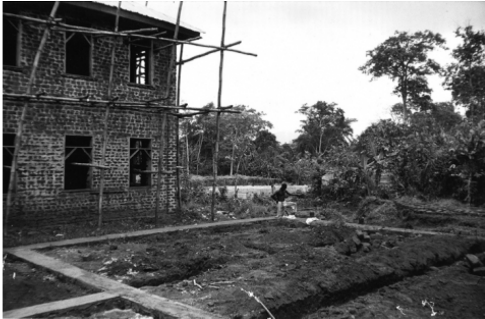
Figure 5 – Foundations of Adesiyan's house next to the one-story building that served as a field office to Willett, January 1958.
