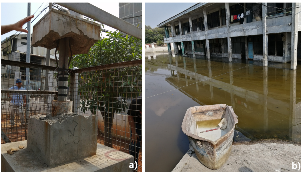
Figure 4. Some local remains of land subsidence: (a) damaged deep pile benchmark installed in 2009; (b) flooded apartment complex.
