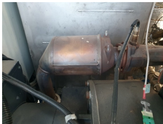
Figure 14. Catalytic converter for CO oxidation.
