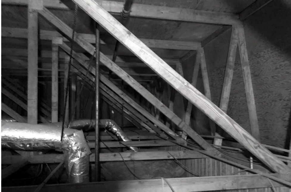
Figure 1.4 Series of repetitive flat roof trusses sitting on the exterior roof wall. Of particular interest is the unbraced 2x4 compression web member running diagonally up from the exterior wall.
