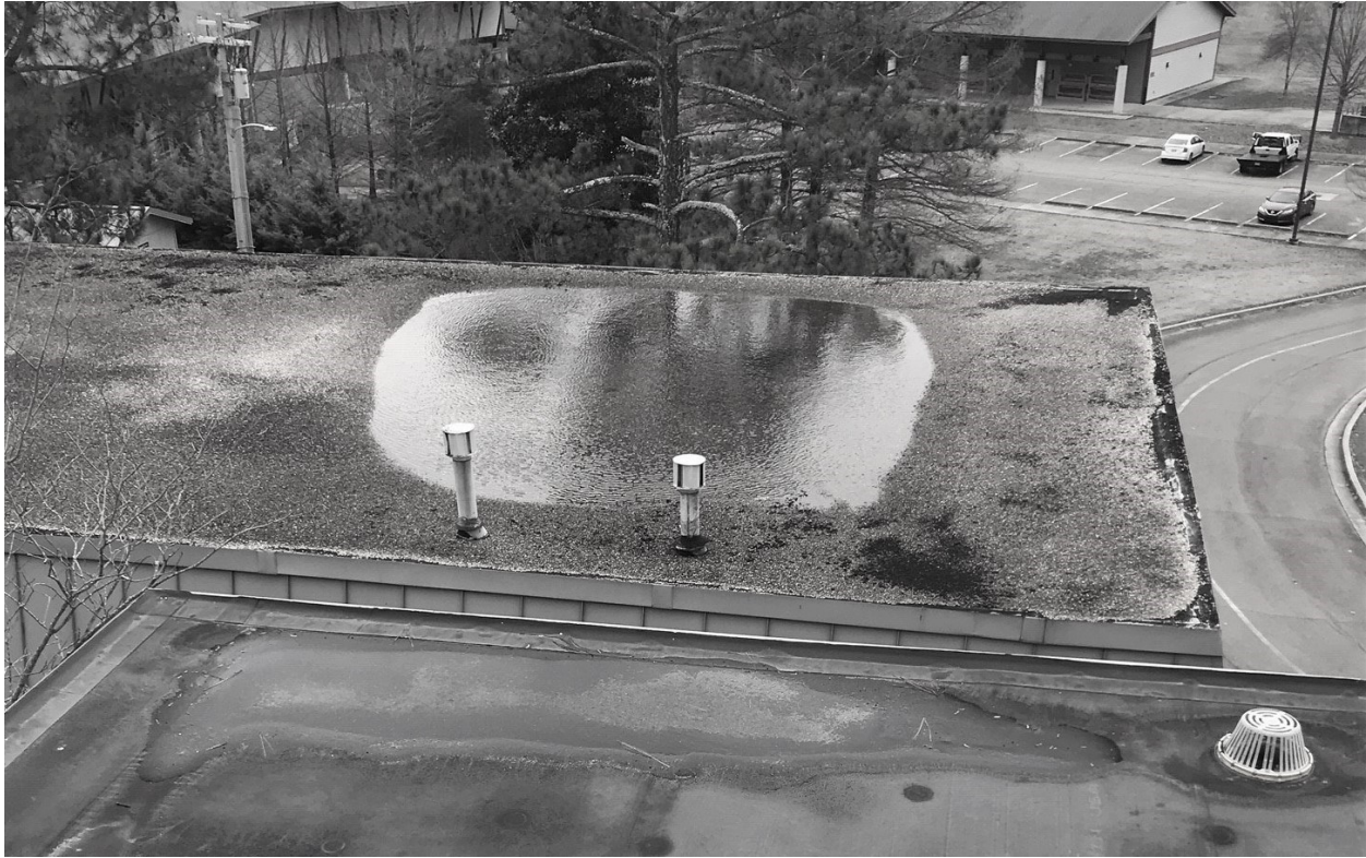
Figure 1.2 Ponding on roof, over an estimated 6.7 x 6.7 meter (22 x 22 foot) area, hours before a heavy rain and windstorm event during which the roof collapsed.
