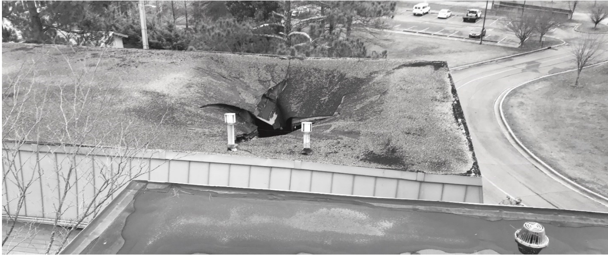
Figure 1.3 Roof section, approximately 7.3 x 8.5 meters (24 x 28 feet), (7 trusses each 28 feet long) immediately following collapse.
