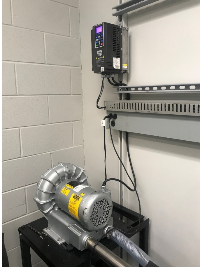
Figure 3.7 1.5 hp Blower and VFD.
