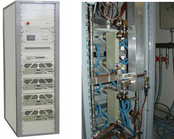
Figure 9: 10 kW cabinet and 6 and 10 kW hybrid combiners.
