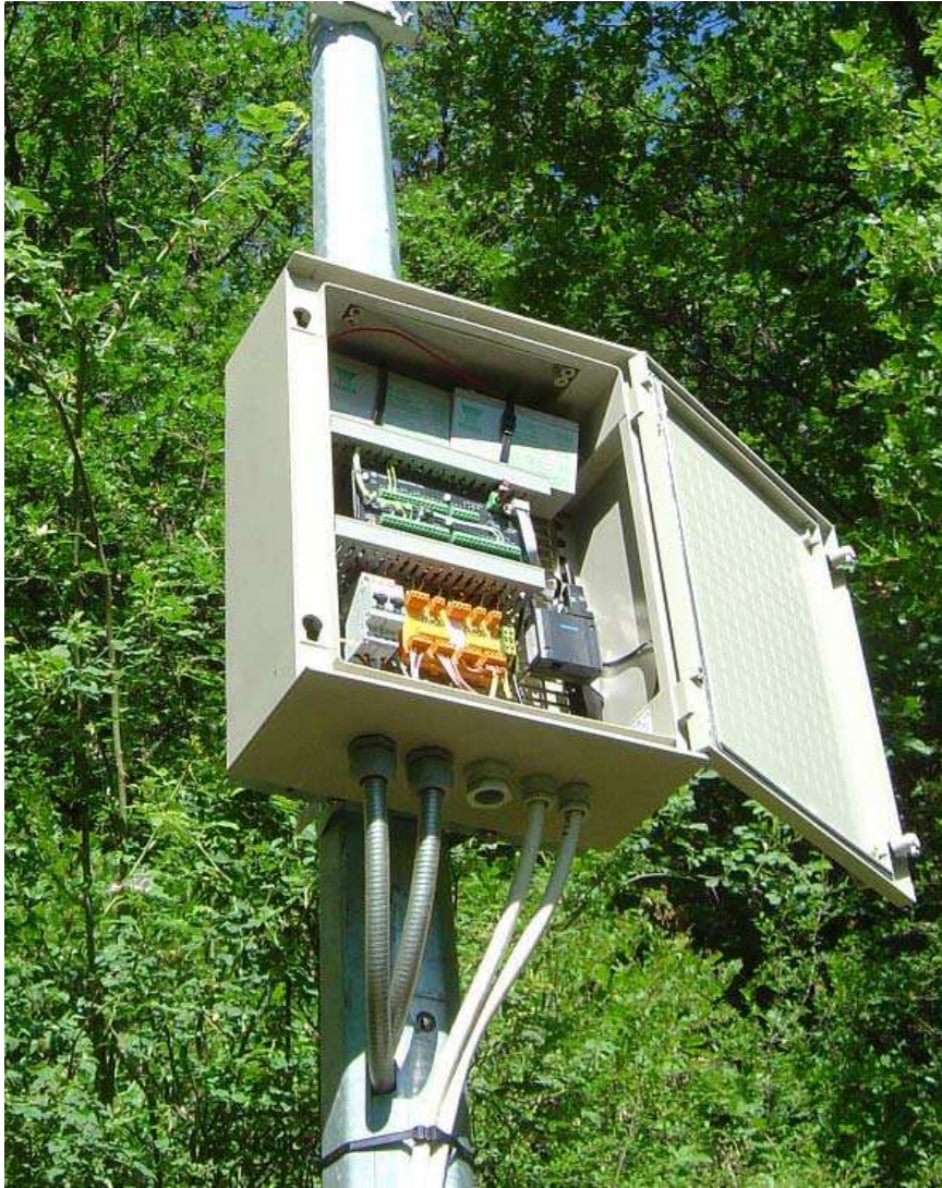
Figure 7. Box that protects electrical and electronic elements.
