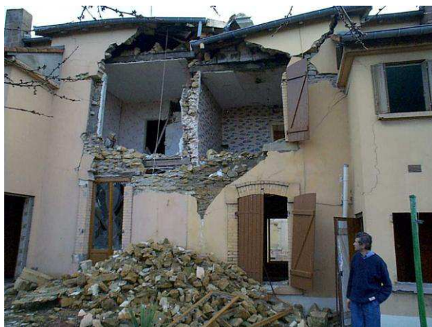
Figure 2. Damages generated by the Auboué subsidence event.
