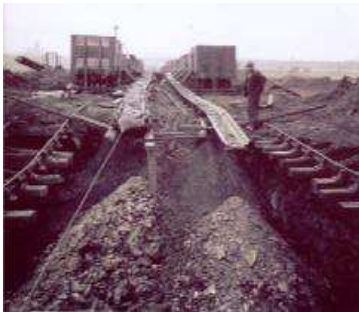
Figure 4 : Infilling Shaft Post Collapse (Source: MRSL)
