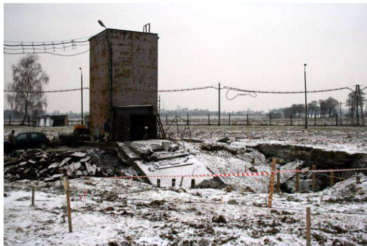
Figure 6 : The crater in the neighborhood of shaft “V” (Source: GIG / KWSA)
