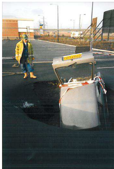
Figure 2 : Collapse of ground in the car park area (Source: UK Coal Authority)
