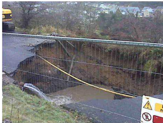
Figure 5: the collapsed shaft at road between Brithdir and Tirphil (Source: UK Coal Authority)
