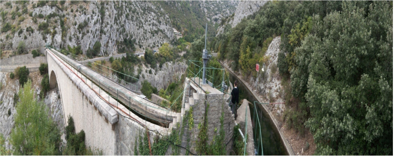
(a) The right bank (RB) and the left bank (LB) of the canal at Partiteur station.
