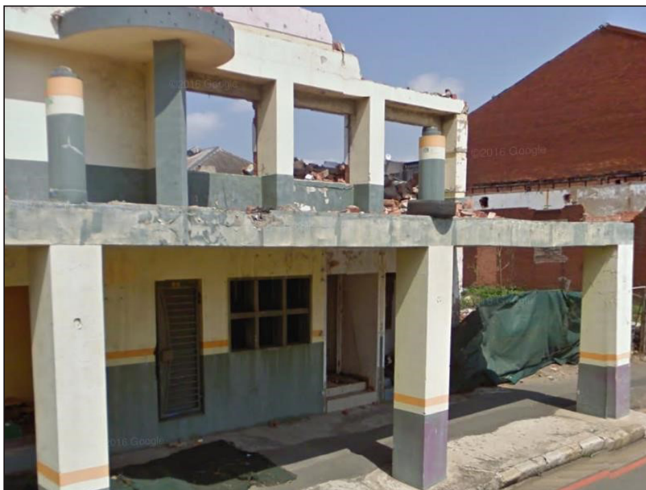
Figure 6: Physical decline evidenced by dilapidated buildings.
