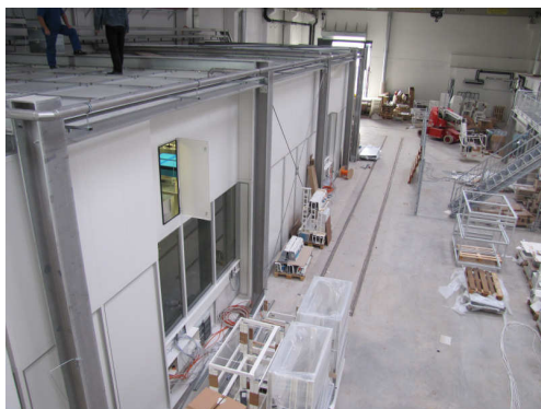
Figure 3: Exterior top- and sideview of the clean room: The outer casing is complete, while the installations inside are ongoing (see Fig. 4).
