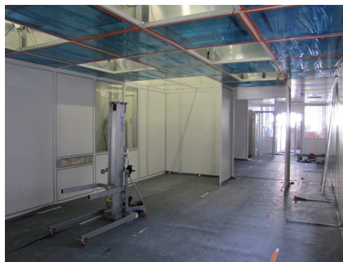
Figure 4: View inside of the clean room (same direction as in Fig. 3), from the ISO 4 area facing towards the ISO 6 and the air-lock area: The double floor is completed, while the installation of the filter-fan units, plumbing and electric installations is ongoing.
