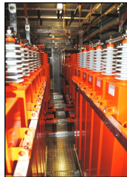
Figure 2: New power grid filter for SIS18.
