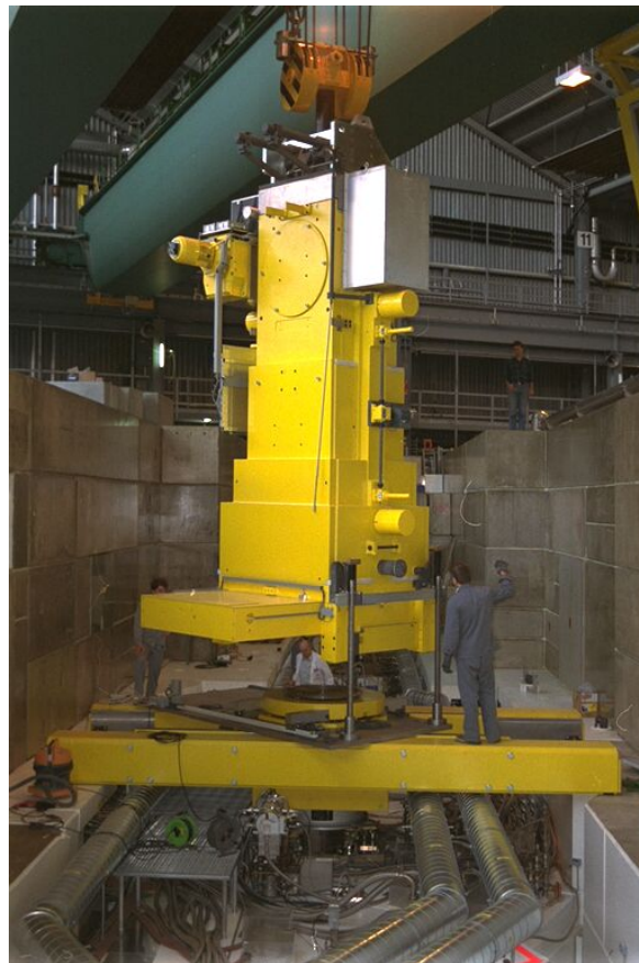
Figure 63: Radiation shielding bottle at PSI [8] to move activated parts to a hot cell. The whole plug is pulled into the bottle which is then transported with a crane.
