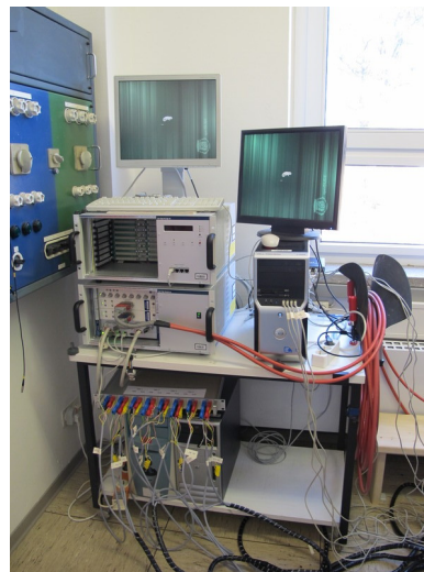
Figure 2: The TRD services infrastructure with the Mpod mini crate visible in the middle left part of the picture
