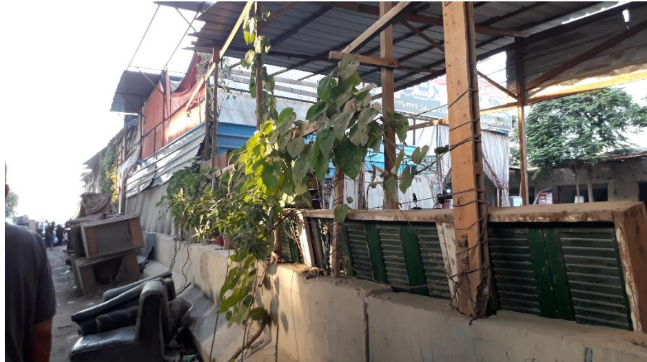
Figure 97- The Growing of Climber Plants on the Crossings of the Wooden Beams (Author's Footage, 2020). Click Here for reaching its location on the keymap.
