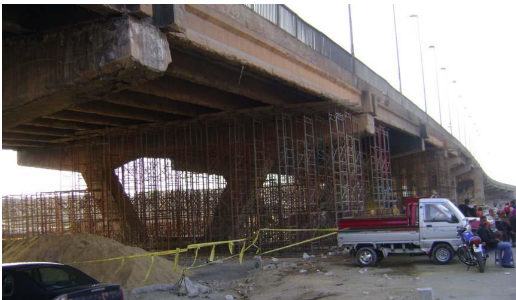
Figure 40-Treating the Construction Problems of the Bridge (Mohamed, 2011)
