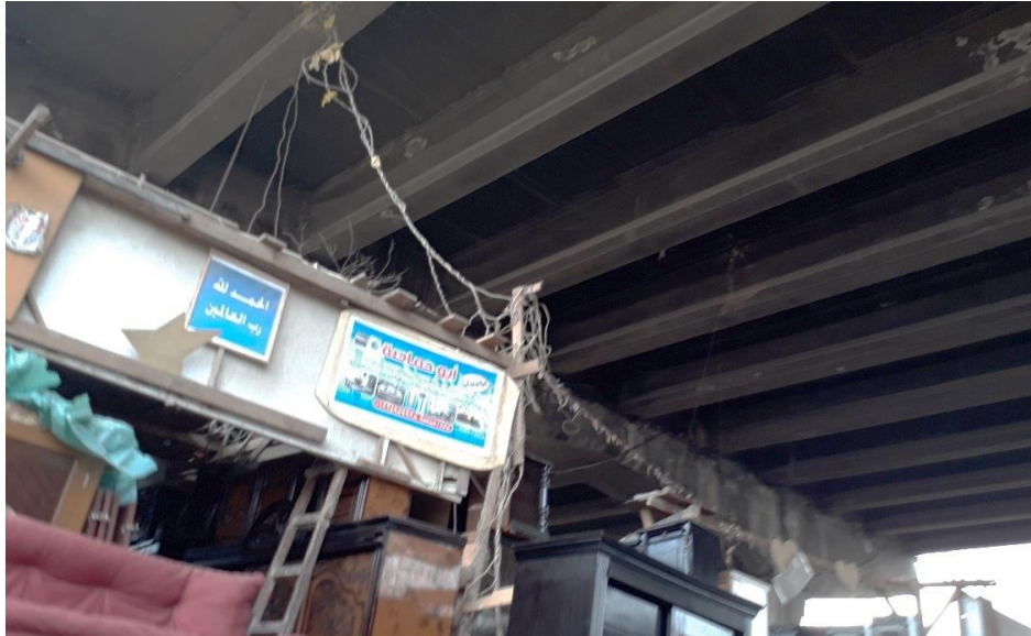
Figure 103- The Hanging of the Pulled Electricity Wires Under the Bridge (Author's Footage, 2020). Click Here for reaching its location on the keymap.
