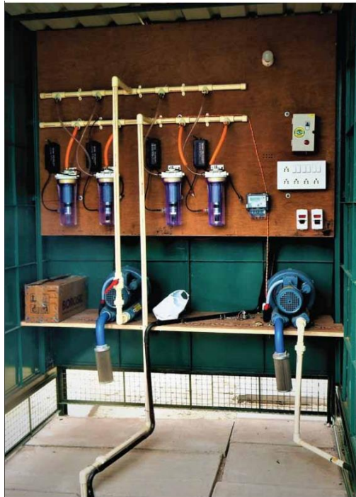
Figure 9. High throughput ozonator in pilot plant.
